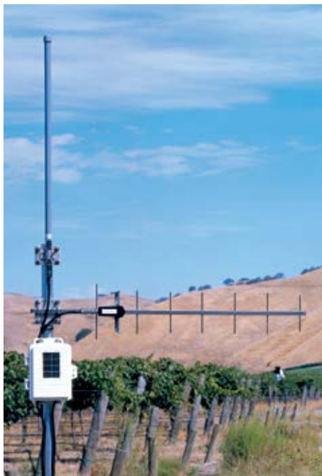
Long-range repeater with one Yagi and one Omni antenna.
