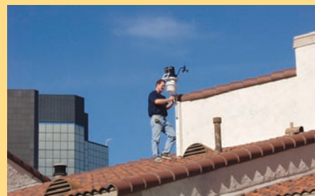
David and Bz Sommers installed a Vantage Pro Plus on the roof of their townhouse in Woodland Hills, California to keep an eye on UV levels and help guard against skin cancer.
